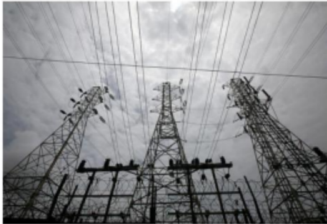
Power struggle: India's peak power demand has been hovering between 230 gigawatts and 250 gigawatts in the past week. REUTERS
